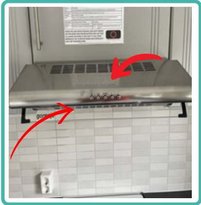
Kitchenfan building A/B/C
