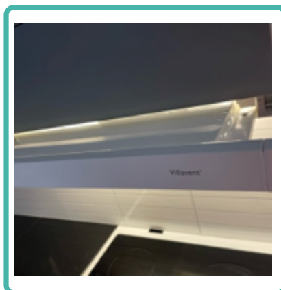
Kitchen fan Meekvegen
